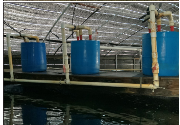
Figure 6. Two different setups showing the combination of degassing units and holding tanks, which could also include biofiltration. At top, pipes take water from the degassing units to the storage tank. At bottom, the water falls directly from the degassing units (blue barrels) into the holding tanks below.
