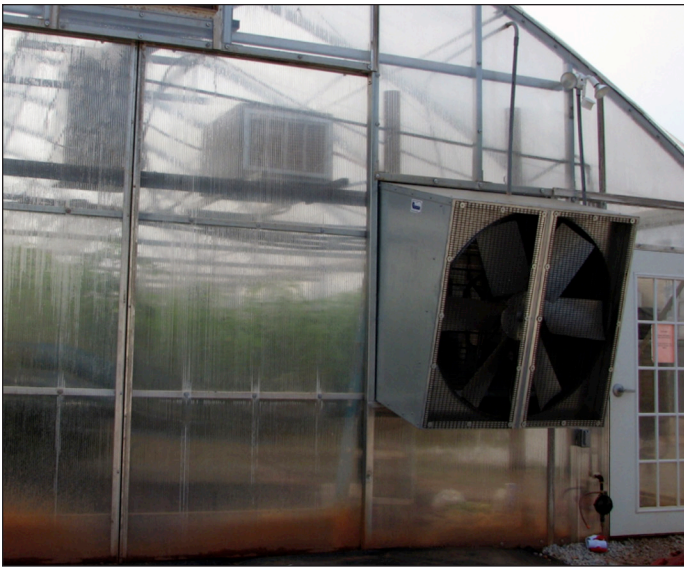
Figure 1. Slant wall exhaust fan.
