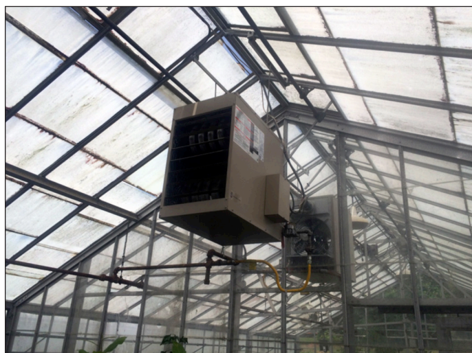
Figure 9. Gas-fired unit heater.
