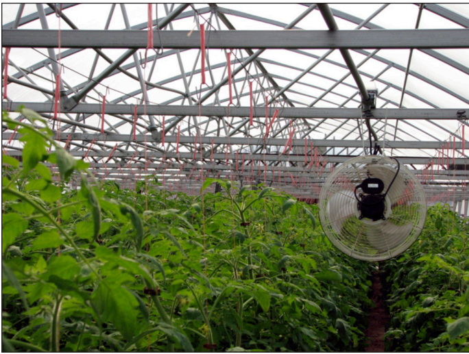
Figure 10. High airflow (HAF) fan.
