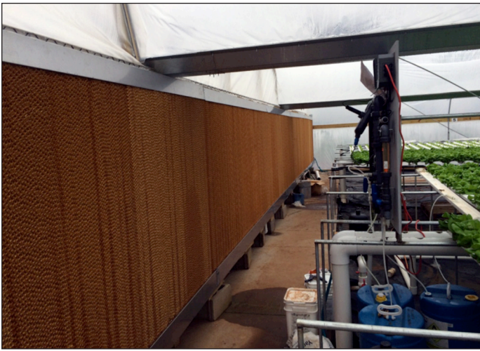
Figure 2. Evaporative cooling pad system.
