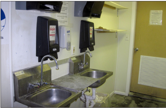
Figure 4. Hand washing station.
