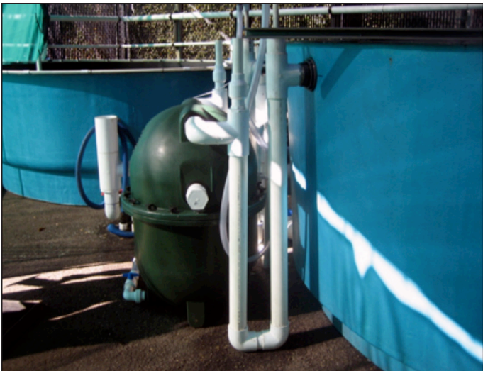
Figure 8: RAS treatment does not have to be complex. This marine fingerling system is supported by a floating bead clarifier and a set of airlifts.
